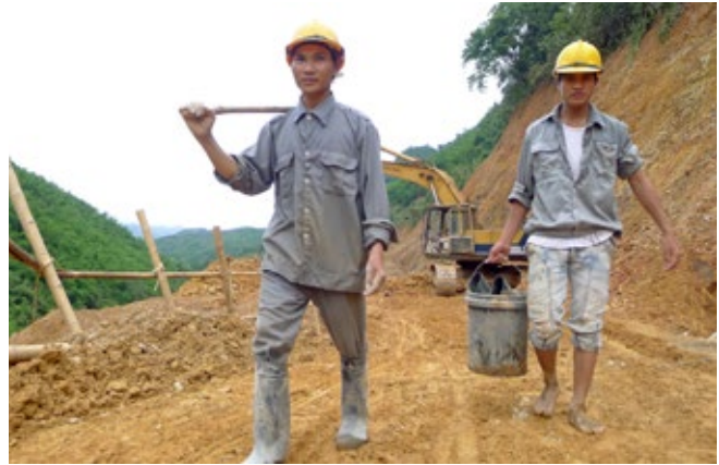
Trung Son Hydropower Project, construction site, Mai Chau, Viet Nam. Photo: © Mai Ky for the World Bank
